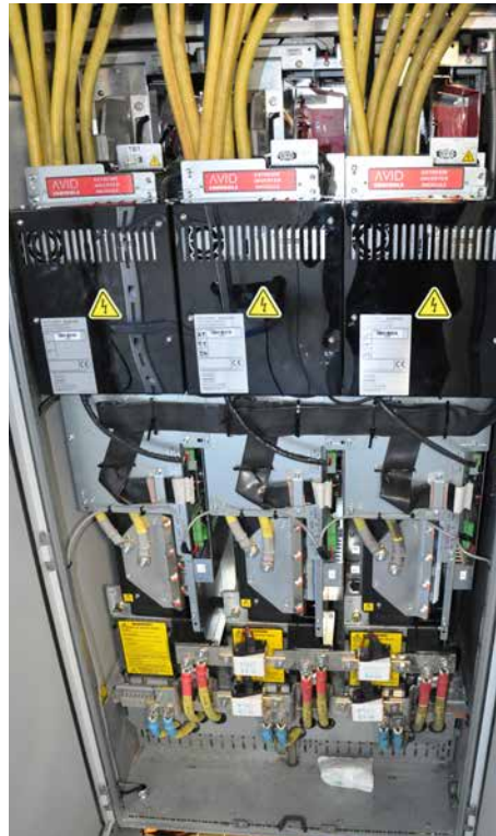
New AEI Retrofit Kit Inverter System Installed
