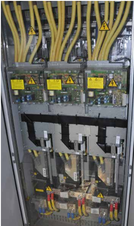
Old Existing Delta Inverter System
