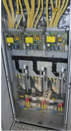
Old Existing Delta Inverter System
