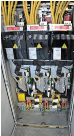
New AEI Retrofit Kit Inverter System Installed
